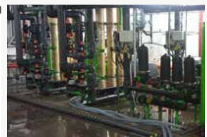
AZUD HELIX AUTOMATIC 203 AA Centro spa y fitness Holmes-Place
